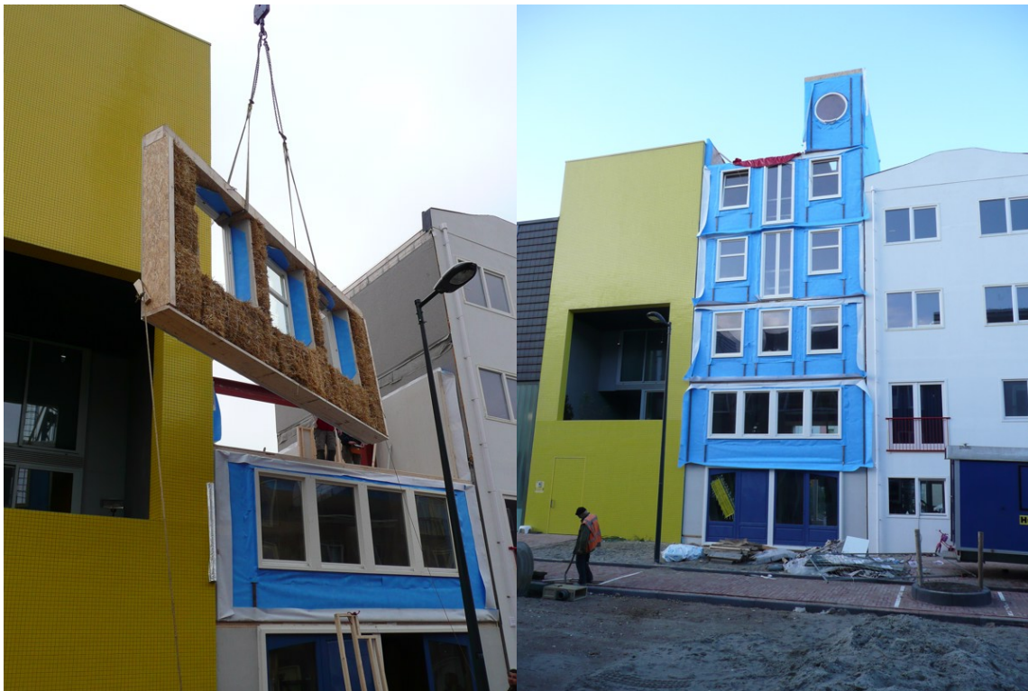
Figure 16: 5 Story Precast Straw Bale Structure in The Netherlands Courtesy of: Rene Dalmeijer
